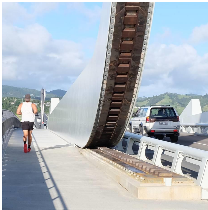
Figure 48: Example of a rolling track located between footway and carriageway unlike the reference design for the Scheme where it is placed on the outer edges of the bridge deck
